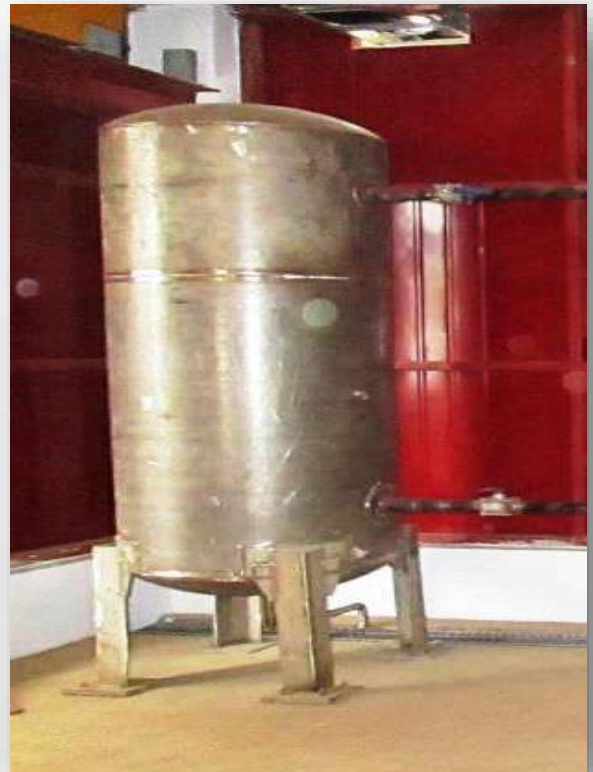
COMPRESS AIR TANK
