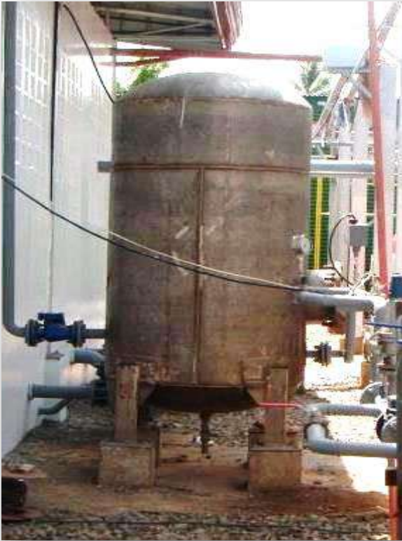
RAW WATER PRESSURE TANK
