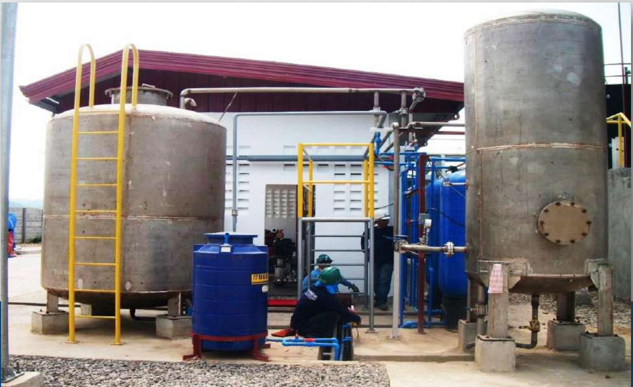
SOFTWATER STORAGE TANKS
